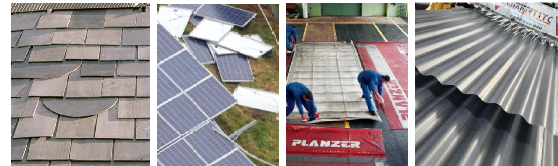
Lightweight and waterproof roof. The cladding can vary depending on the available resources. wood, (disfunctional) solar pannels, truck tarp, metallic sheet...
