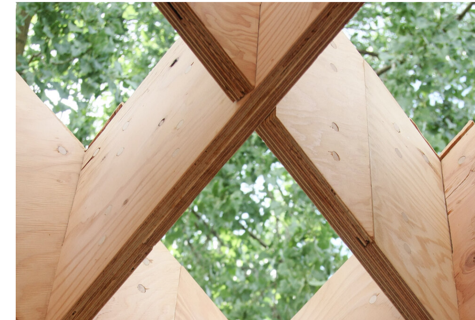
Example of plywood joinery with dowel joints. Sidewalk citizen solarium, Studio North. Double layer plywood connected with dowel joints, to form the joined shape of the structure.
