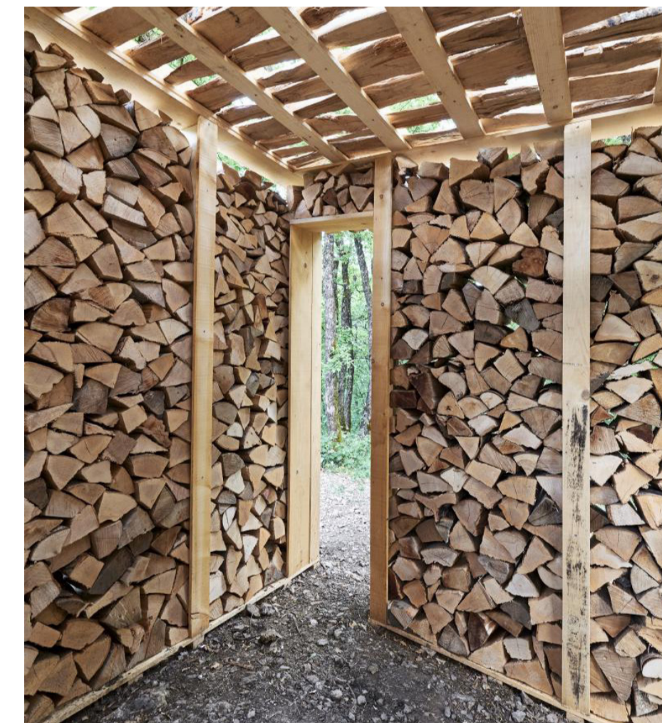
Pavilion constructed from fillings of oak firewood / Louis Cayol and Angela Aguilera
