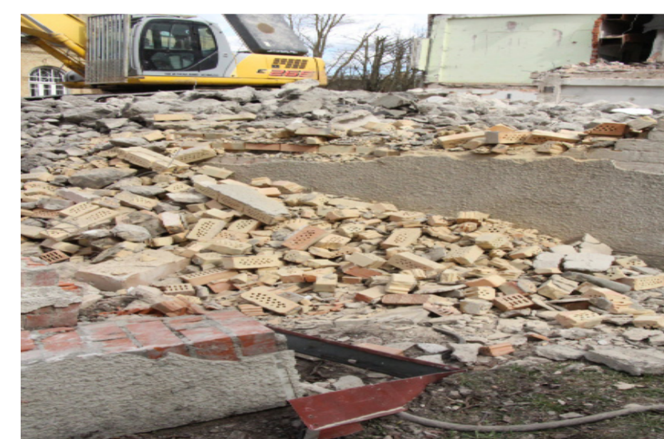
Construction debris used as foundation – picture by the authors
