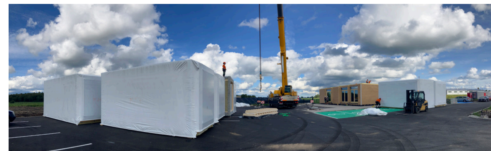
Wrapping foil on a CLT building site in Estonia – picture by the authors
