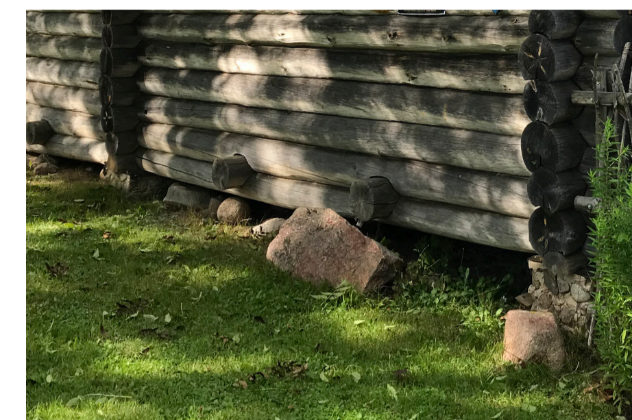
Traditional foundation of a log house in Latvia (national heritage) – picture by Juris Dambis
